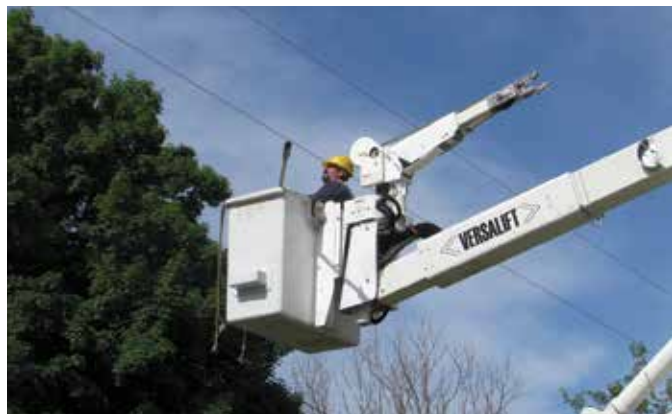
Jason Walter grounds overhead lines to prevent shock when the linemen work on the line.
