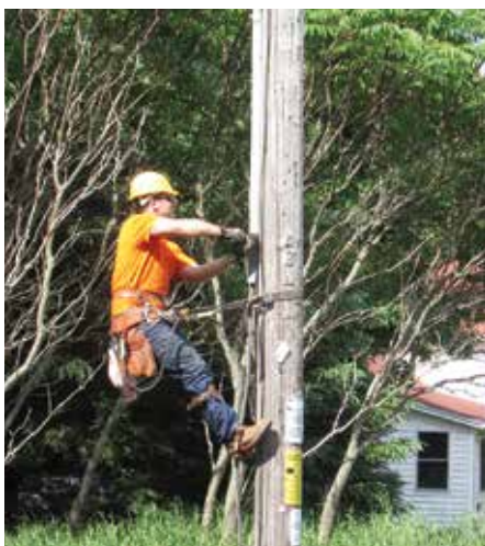
Gabe Pospyhalla climbs an electric pole via harness in order to remove guards that protect cables and wires from the elements.
