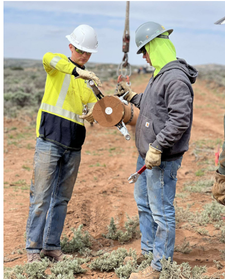
Alex Lutz (left) spent a week in Arizona helping install power poles to bring electricity to residents of the Navajo Nation.
